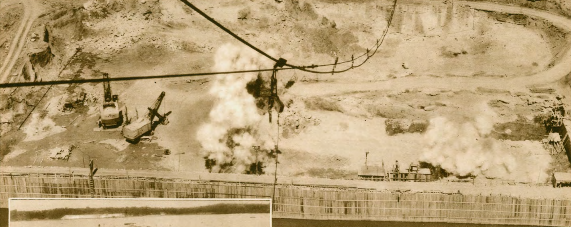
ON THE CLINCH RIVER, four hundred miles up-stream from Wilson Dam, is the site of Norris Dam — now under construction by the Tennessee Valley Authority. Primarily a storage dam to provide a year-around water supply for dams down-stream, Norris Dam nevertheless will generate 120,000 horsepower. While serving people many hundreds of miles away, this great dam at the same time will make cheap power available to the people of the neighborhood. It will be a major factor in the control of floods.
