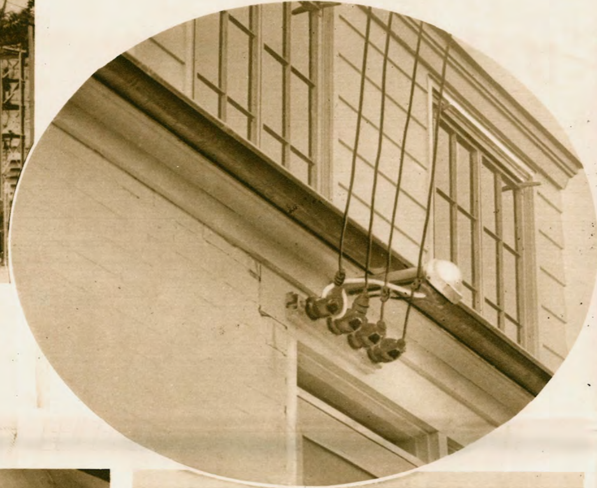
Here is how cheap electricity enters a typical Norris home. Note more wires than usual; electricity is used abundantly in Norris homes to save time and labor in household tasks.
